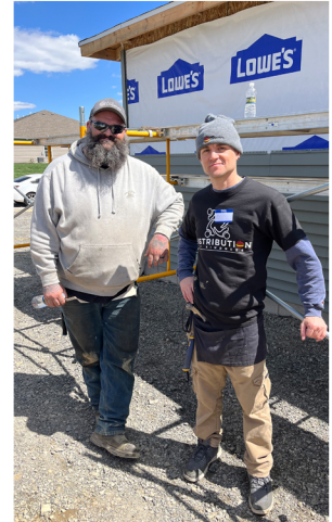
Zach Hall, Eric Baker, and Pam Orwick donated their time to install siding on a new home for Habitat for Humanity.
